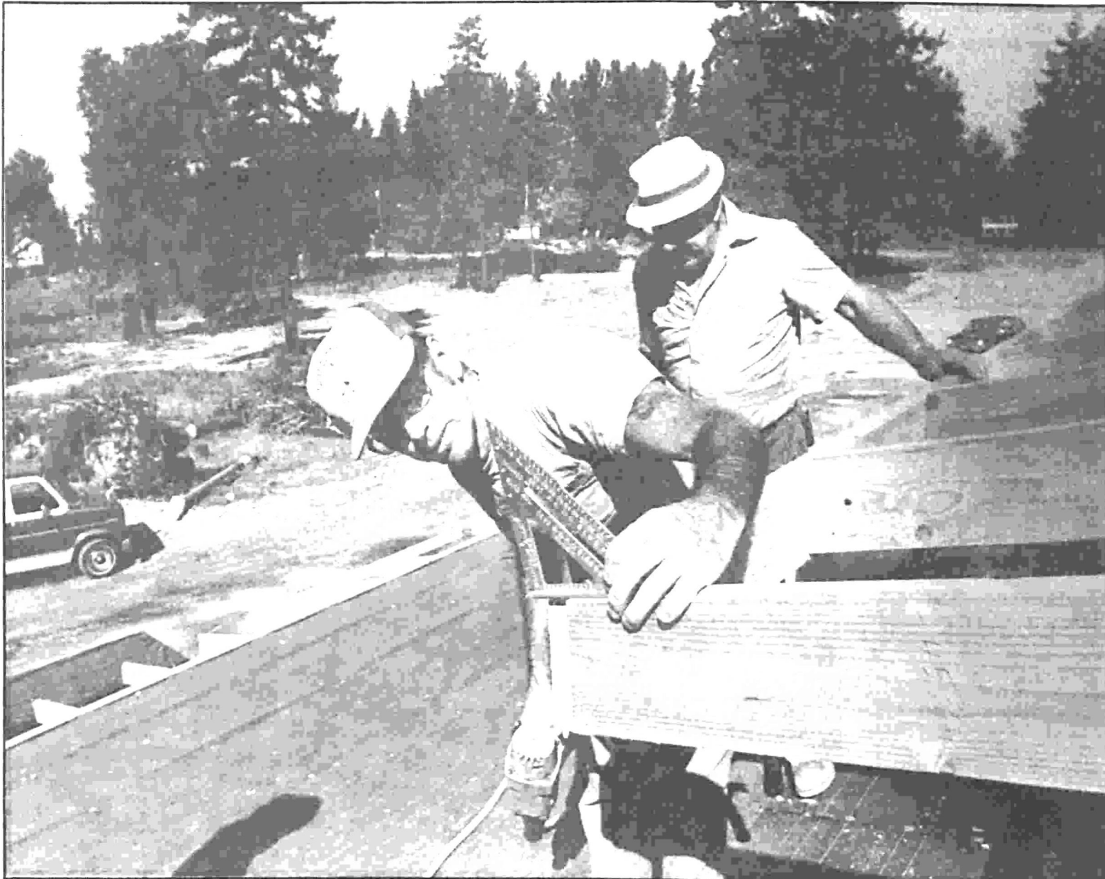
N.I. RICE (front) and Joe Fink get back to work on the roof of the new Baptist Church at Palisades after taking a lunch break. The two Texas natives belong to Volunteer Christian
