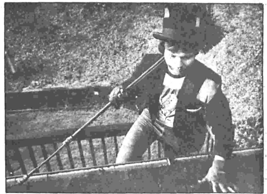
IT CAN AT times be a dangerous profession to crawl on rooftops, especially during the frost-covered mornings. Tom says he loves climbing on roofs because of the great view from that height. And he's only fallen off once.
