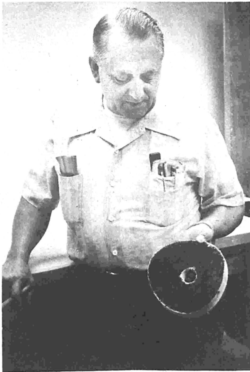
BILL MARTIN, manager of Water District 124, shows evidence of manganese that has settled in some of the district's pipes. This pipe, originally cement white, has been blackened by the mineral found in the well water. Martin said the district plans to begin pipe-cleaning procedures within two months to red the district of the black water problem caused by the manganese. the problem. Those are the Twin the problem is recognized in Lakes and Camelot areas. other regions of the district, they Martin said, however, that if also will be flushed.
