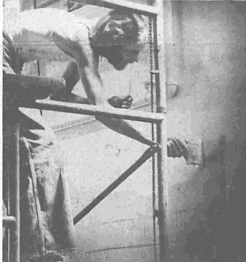
REPAINTING THE walls of the gymnasium at Federal Way High School is one of the many projects underway as the local school district catches up on long-overdue maintenance. The painter is Tim McCarthy of Federal Way, a member of the district's newly hired crew of trainees.
